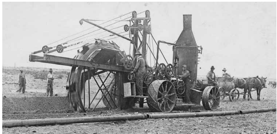
Men laying the water mains in Camp Cody using a steam-driven trenching machine. Deming-Luna Mimbres Museum Archive
