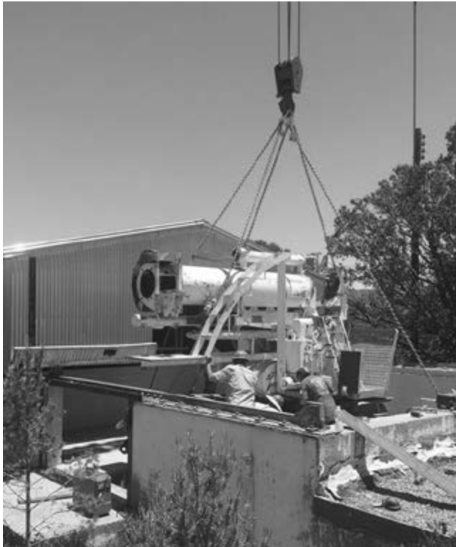
T4 being lifted by 75-ton crane at Mule Peak site in 2019. Notice retracted roof of shelter building. Photo by Phil Esser.
