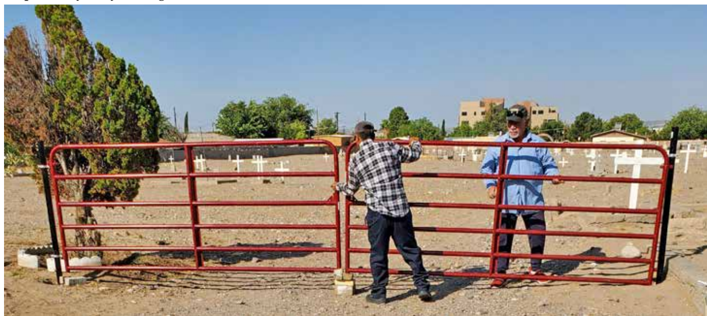
Cemetery volunteers Jose and Albert get the inner gate lined up during installation on Aug. 21, 2023.
